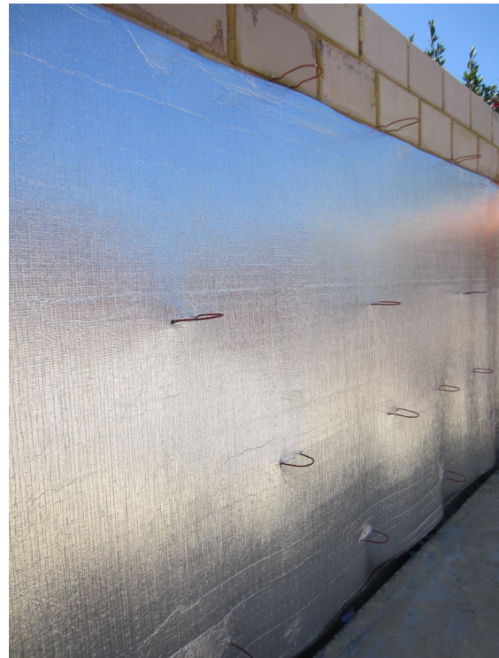
Reflective insulation (photo by Josh Byrne)
